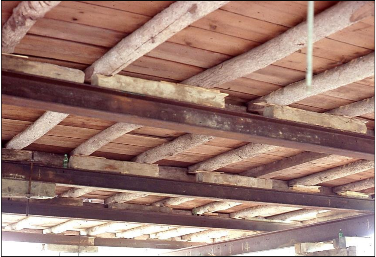
First floor frame, camera facing northeast, June 1979. The east-west floor girders support the ends of rounded sleepers. The steel beams were inserted temporarily during the lifting of the building. Photograph by James L. Garvin.
