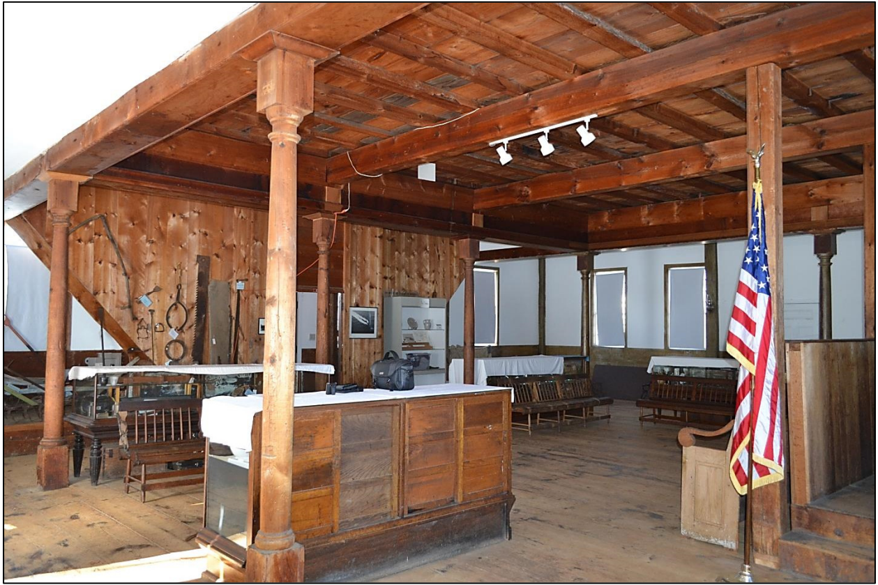
Webster Meeting House: Town Hall on first story, showing original gallery columns and staircase enclosure (rear). Camera facing northwest.
