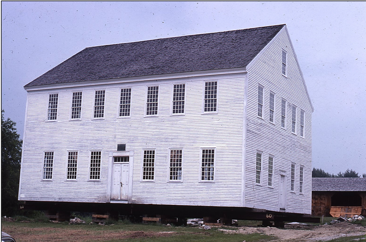
Temporary jacking of the meeting house in 1979 for the construction of a concrete foundation below grade. Photograph by James L. Garvin, June 1979.
