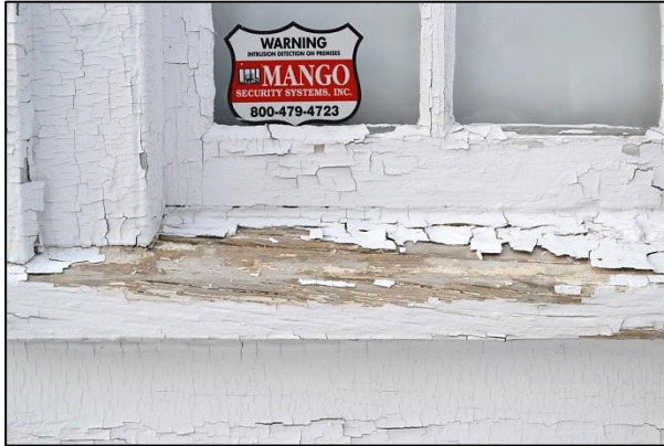
Left: Cracked or checked window sill, south side of building.
